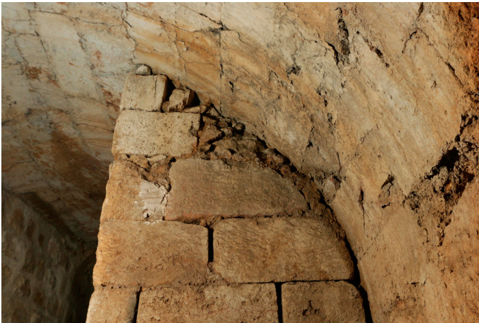
Figure 22. Photo of the first buttress against the south wall of the original chamber.
