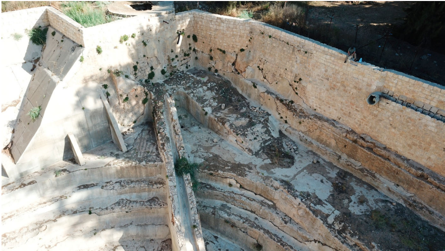
Figure 11. Photo of northwestern corner of the Lower Pool. Note the traces of two basins (filled with earth) at the top of the sloping channel and the wide staircase.
