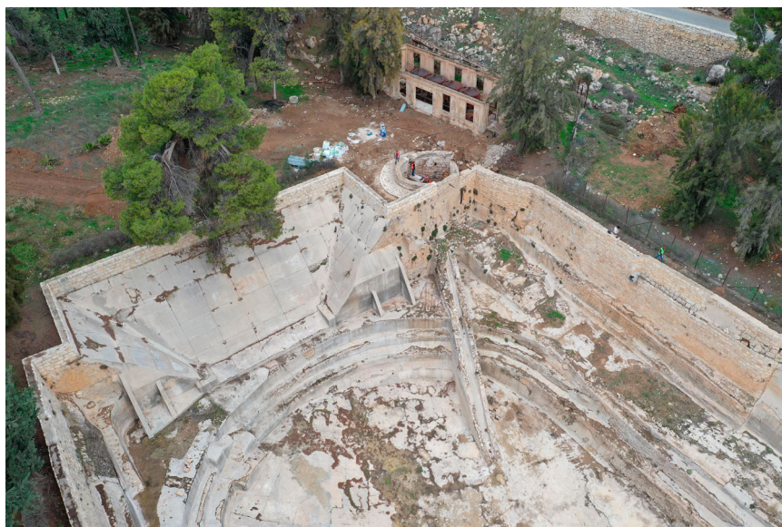
Figure 7. Photo of the northwest corner of the Lower Pool showing examples of the interior terraces of the pool. The large portion of the South Wall that is part of the British Mandate renovation. Note the sloping channel into the pool at centre.
