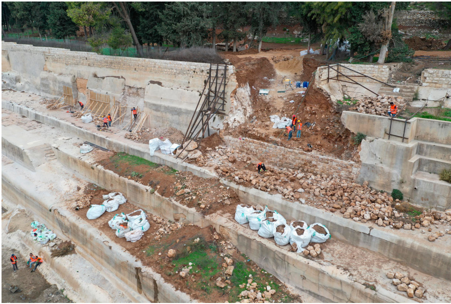
Figure 14. Photo of break in the North Wall of the Lower Pool after cleaning showing ongoing reconstruction work at the site.
