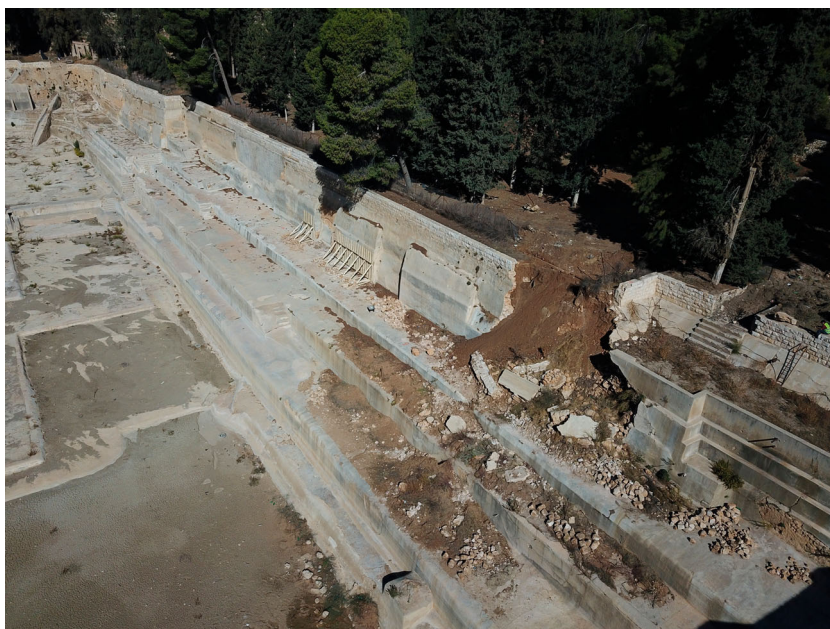
Figure 6. Photo of the collapsed portion of the North Wall of the Lower Pool.
