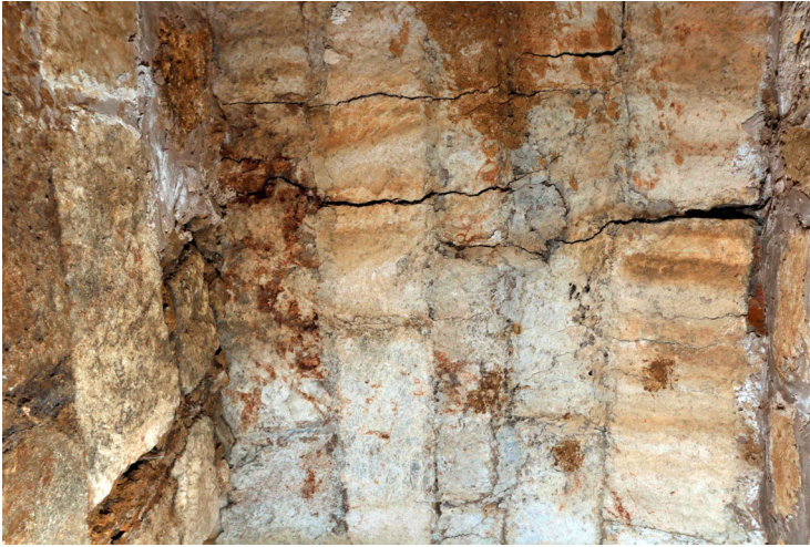
Figure 21. Photo of cracked ceiling within the interior chamber.
