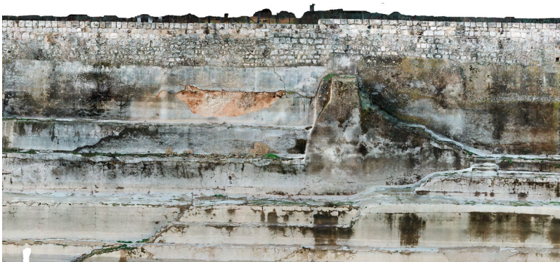
Figure 9. Orthophoto of the Southern Wall of the Lower Pool, showing collapsed plaster due to the buckling of the wall above. Collapsed plaster reveals bedrock with upper retaining wall. Note bedrock staircase cut off at centre right. The upper two courses of wall are of relatively recent vintage (ca. Medieval-modern).
